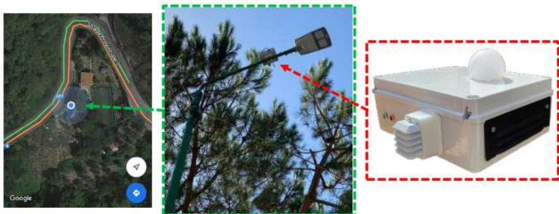
Figure 5.15: Installation and details of the monitoring system.
