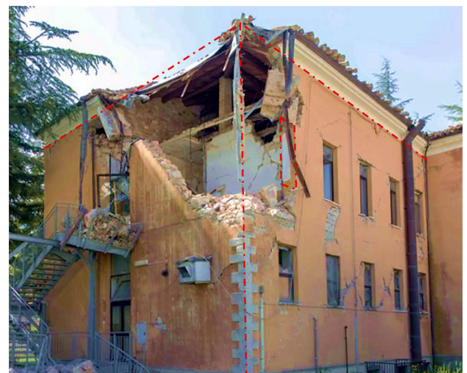
Fig. 11. Out-of-plane failure mechanism of the north corner of the primary school in Visso (Macerata, Italy).
