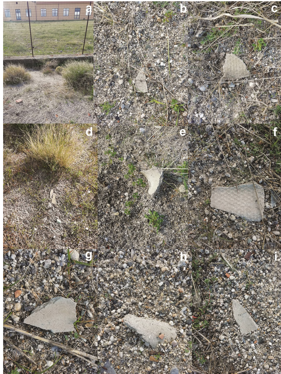
Figure 17. Illegally abandoned ACMs (a–i), located behind the sand dunes exposed on the left side of the Canal degli Inglesi (Lat.: 38°16′18.96″ N, Long.: 15°38′8.98″ E). Source: Authors.
