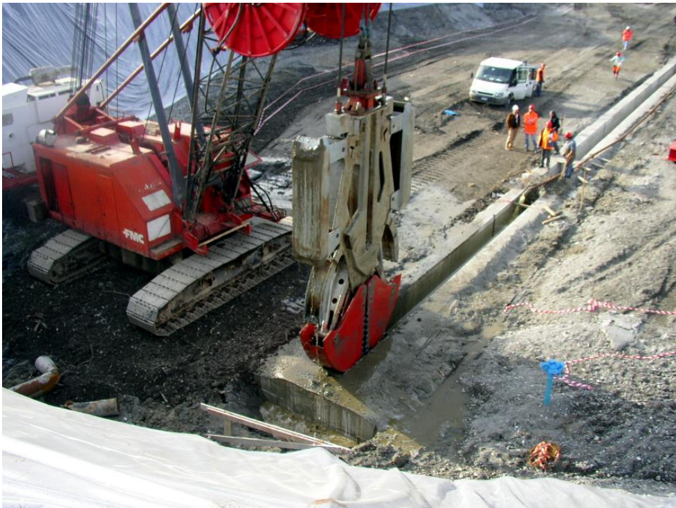
Figure 1.16 Crawler crane equipped and Hydraulic grab used in the excavation of a PRB in Avigliana and Buttigliera Alta (TO), 2004.
