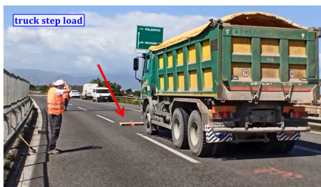
Figure 3.8: Application of an impulsive load by means of the transit of a three-axle truck on a step.
