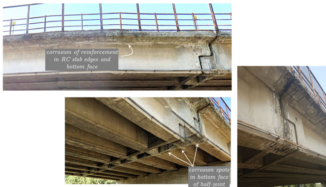
FIGURE 4 Corrosion state localized in the reinforced concrete (RC) slabs (left) and in the half-joints (right) of the analyzed road overpasses.
