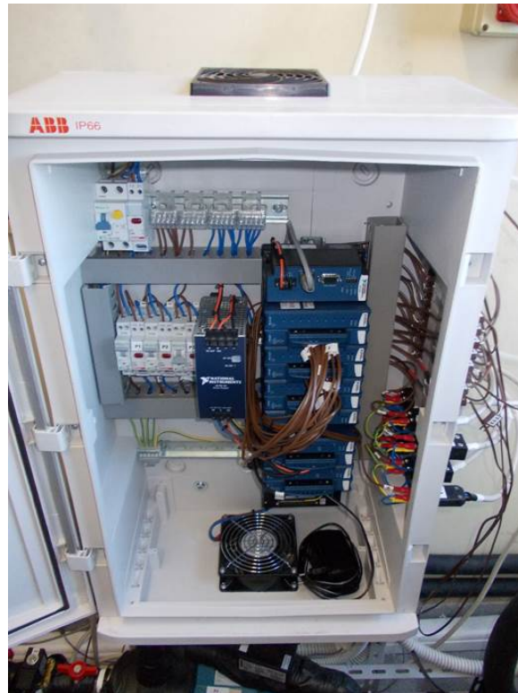
Fig. 3.9 Electric panel and acquisition system of the testing rig.
