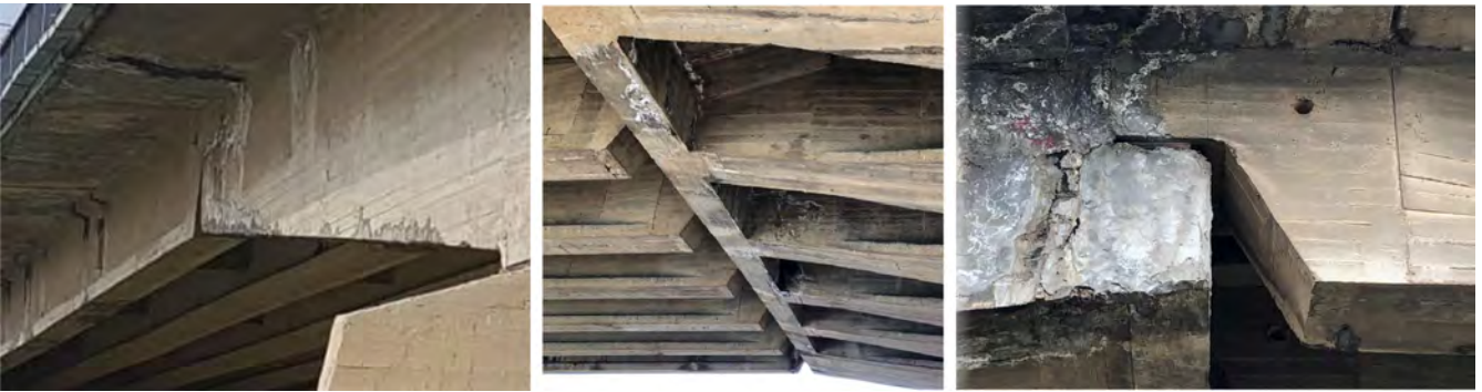
FIGURE 6 Deterioration of the Gerber saddles
