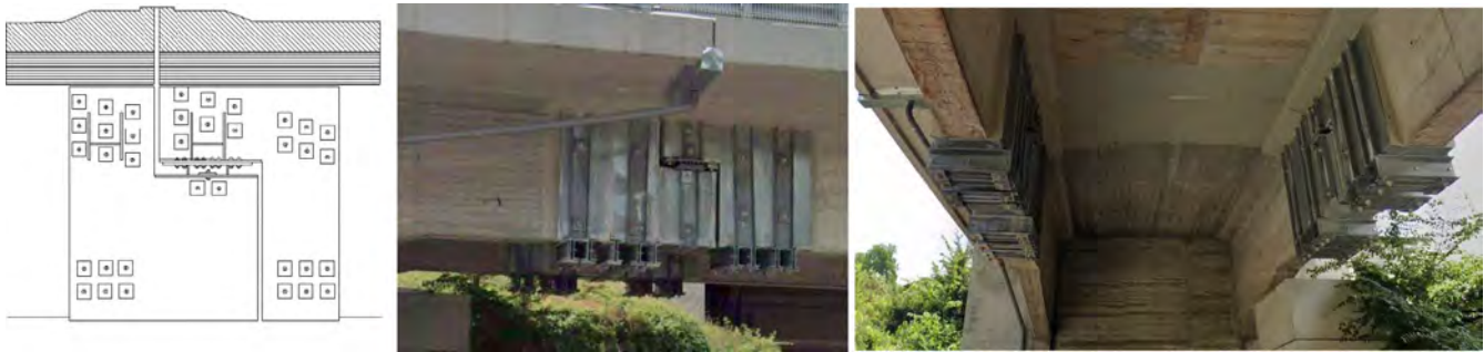
FIGURE 18 Steel plating of Gerber saddles of Sabbione and Generale Franco Romano viaducts (Italy) 12
