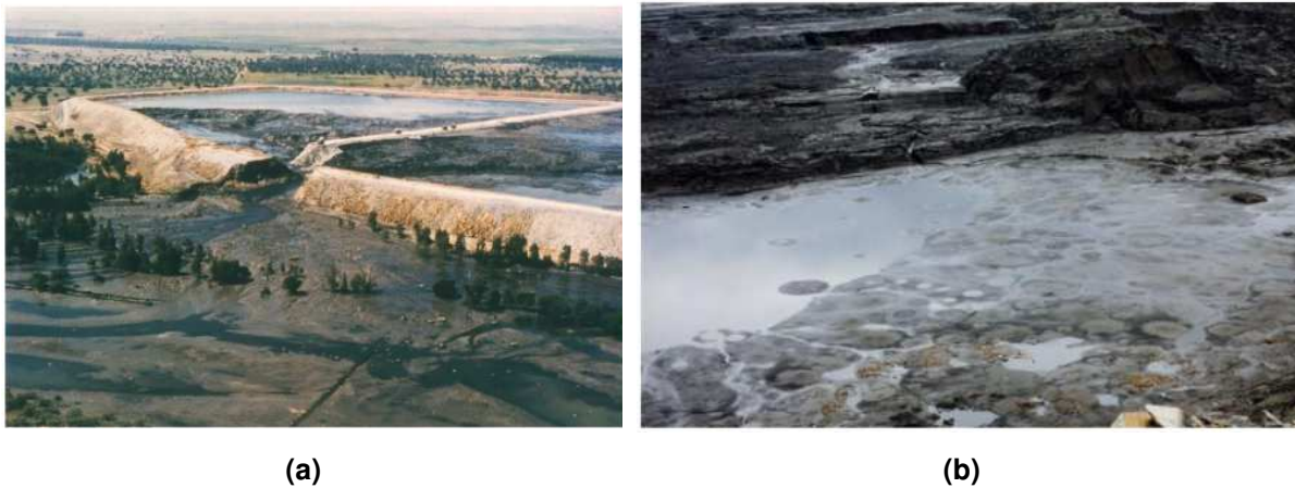
Figure 5 – View of the Aznalcollar dam following the collapse (a) and evidence of the phenomenon of static liquefaction (b) (Gens 2019).
