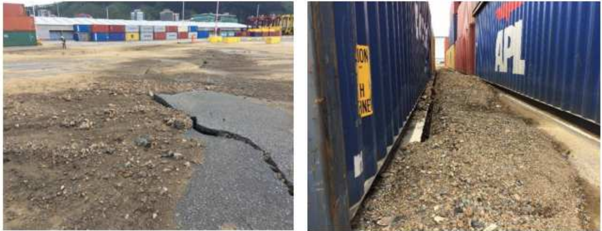
Figure 4 – Manifestations of the phenomenon of liquefaction in the Wellington harbor area following the 2016 Kaikoura earthquake (Cubrinowski et al. 2019).
