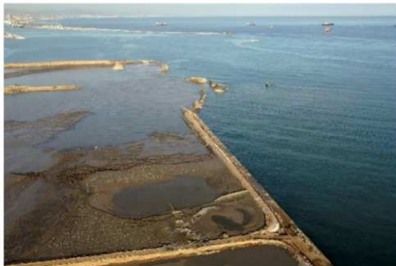
Figure 6 – View of the harbor section of Prat Quay following the collapse (Gens 2019).
